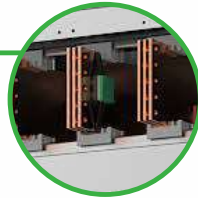
Main Busbar joint
